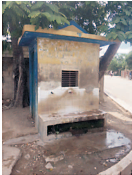
Water kiosk connected to water system they were mapping.
